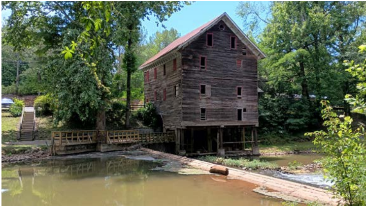
This is a picture of the back of the mill. You will note that there is no water wheel. The mill was powered by water turbines which were underneath the building.
